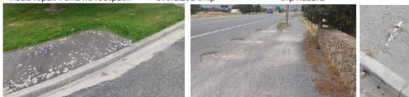
No crossing ramp, path just ends
