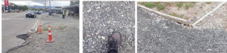
Road repair? and no footpath
